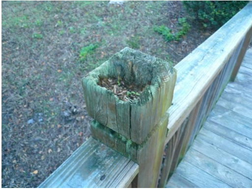
Deteriorated wood on decorative rails and footbridge
