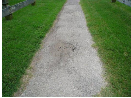
Potholes on asphalt paths as well as root damage
